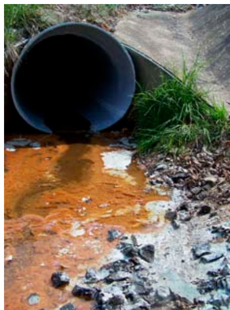
Photo 2. Uncured resin waste (gray substance adjacent to outlet and along rocks on right side of image), 1 week after installation
